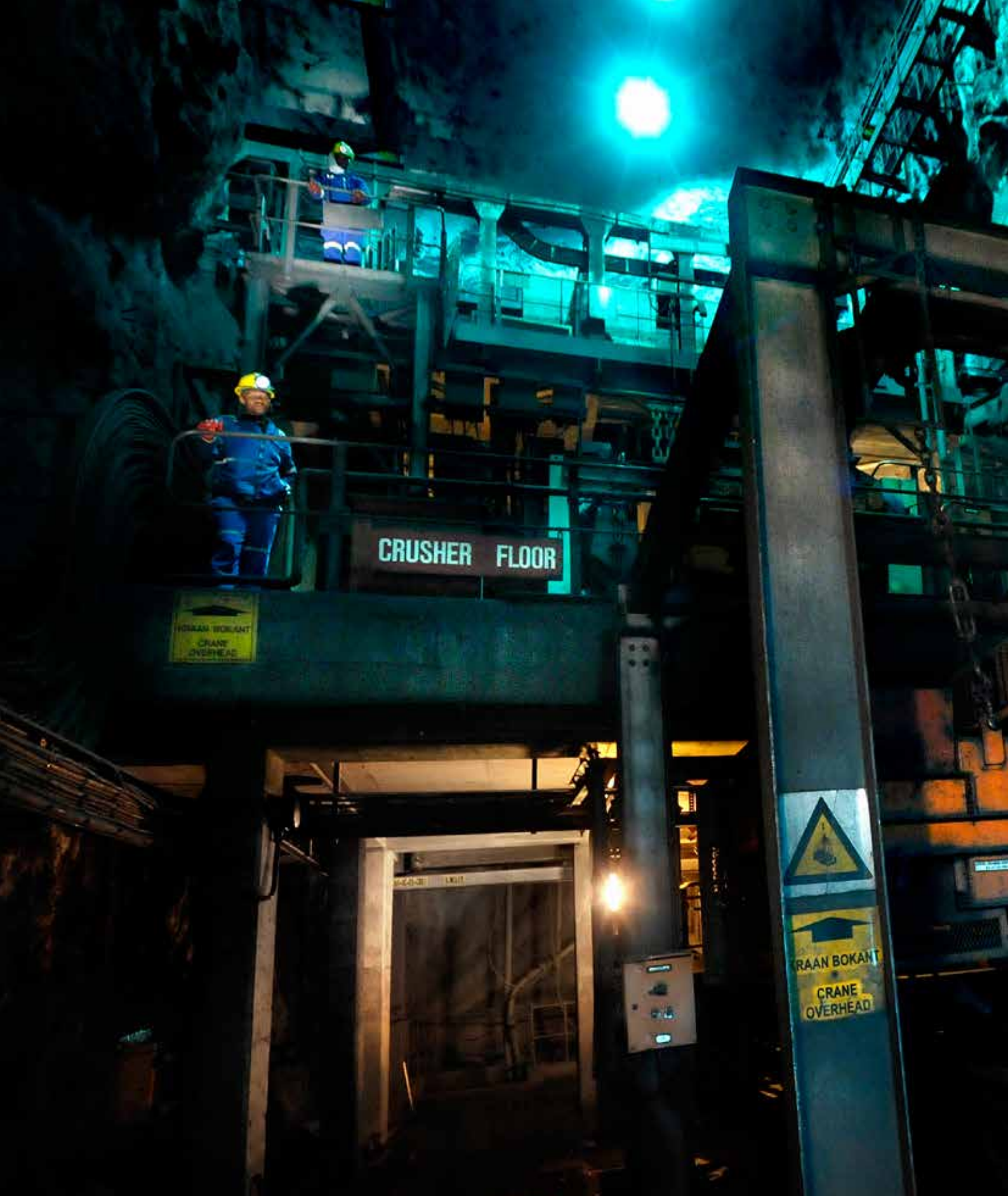
Underground crusher load-out facility at Black Rock Manganese Mine
