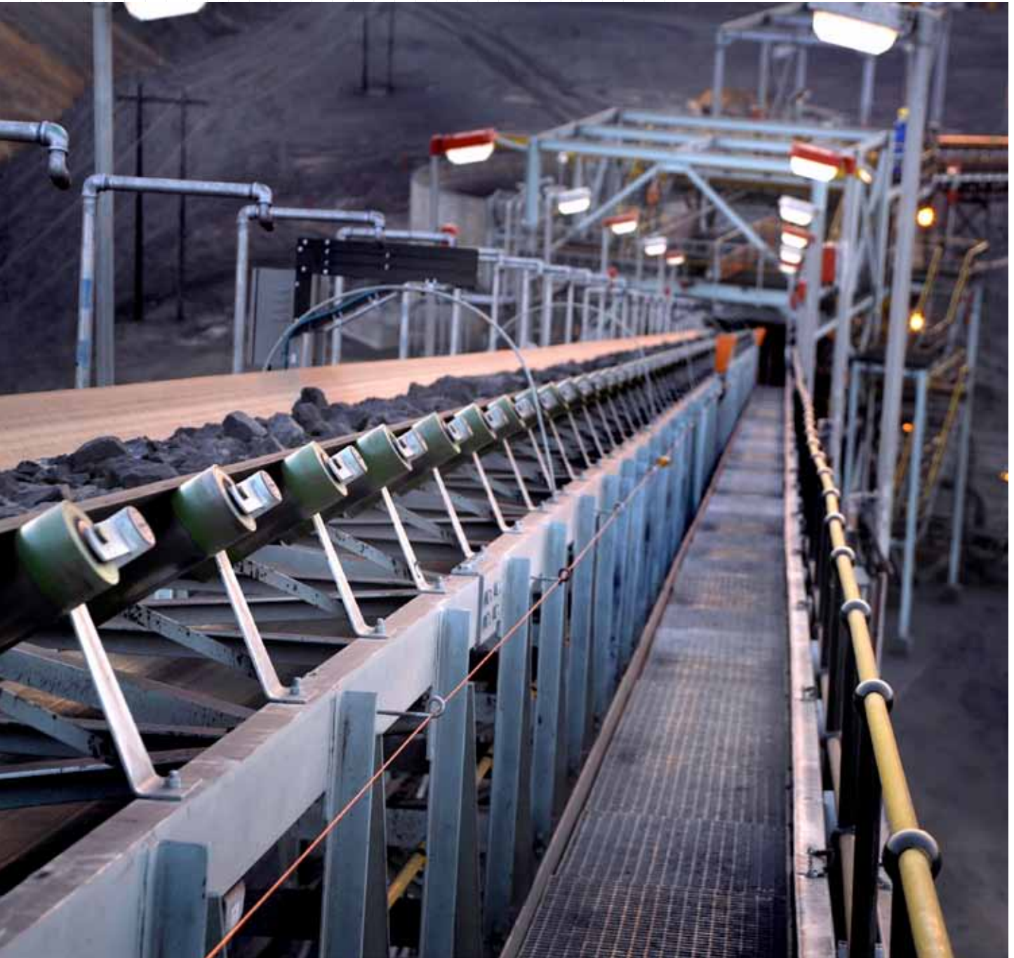
Manganese beneficiation plant at Nchwang Mine.
